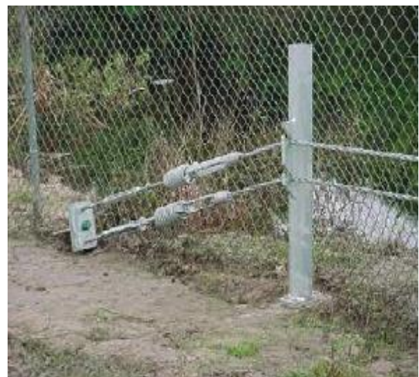
Fig. (3). Heavy-duty springs that anchor cables at the end of the cable barrier segment (used with permission, American Consulting Professionals).
