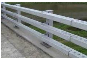
Box beam barrier
