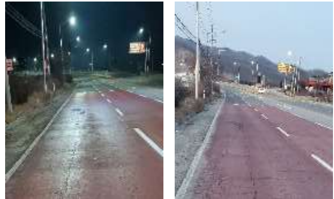
Fig. (1). Pavement with frost (left) and without frost (right).
