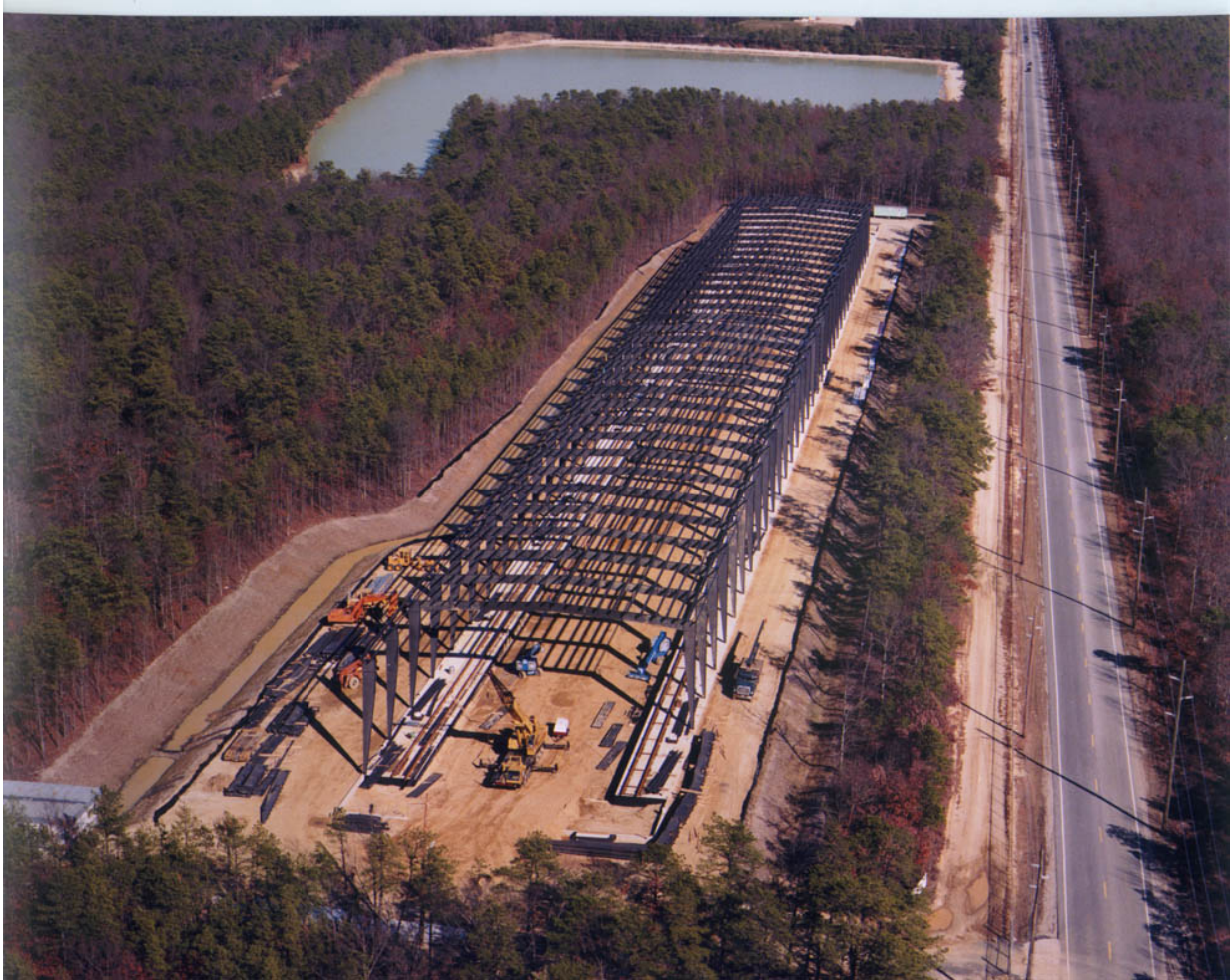
Fig. (1). Aerial view of NAPTF facility under construction (Photo Courtesy of NAPTF)
